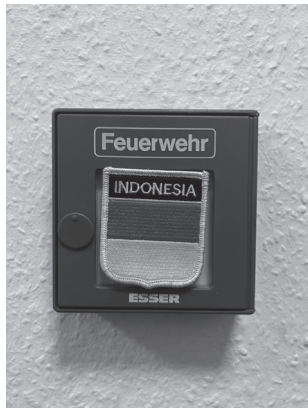
img 10 The fire alarm button at the Hübner factory/JaF house, covered with an "Indonesia" badge. Photo by Simon Kentgens
