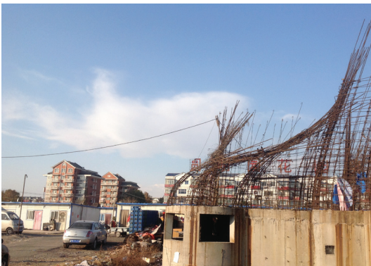
Figure 40. Steel bars protruding from unfinished villas, 2014. Photograph courtesy of Ma Lijiao.
